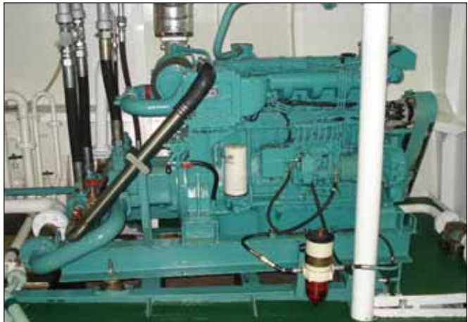
Doosan AD126TI power pack installed in MT "Kintore"
